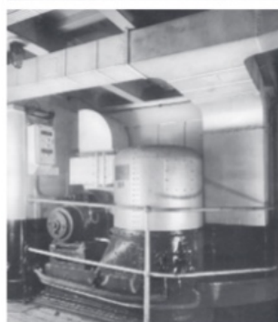
At bottom is a 'tween deck type' on the RMS Lusitania. Note the scale of the trunking above and to the side of the Thermotank.
